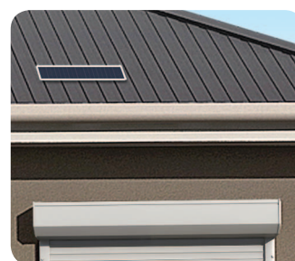
Roof Mounted Solar Panel
